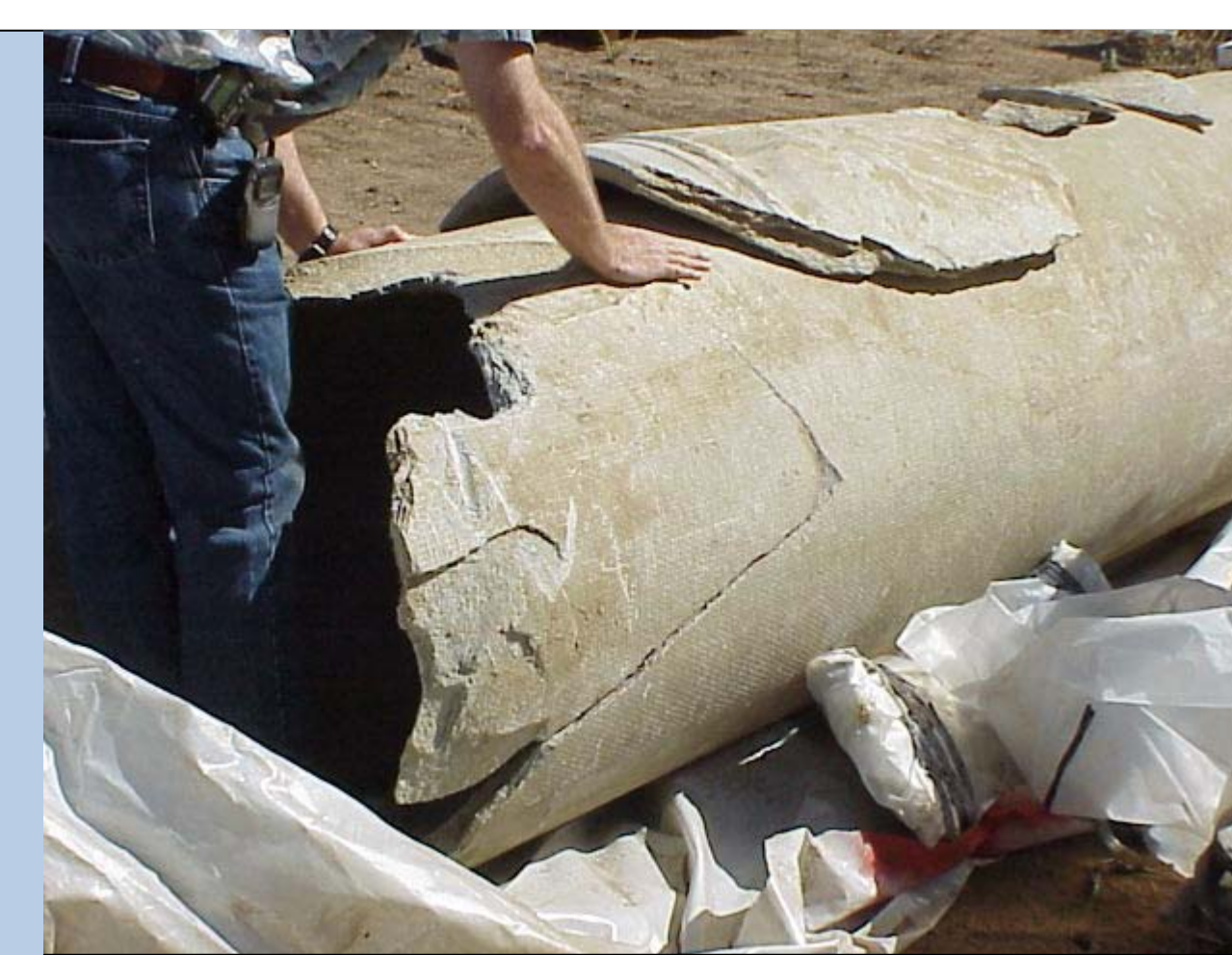
Figure 3. A failed AC pipe (Edwards 2005)
