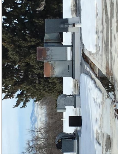
View of Some Mechanical Units
