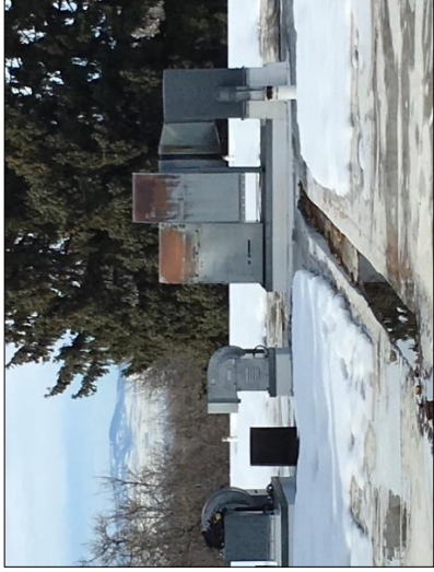
View of Some Mechanical Units
