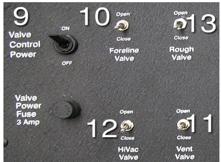
Above: Numbered valve control switches
