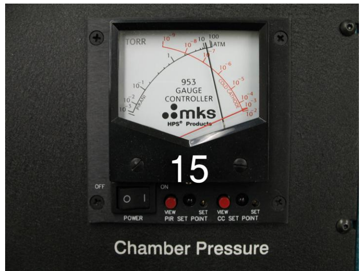
Above: Chamber Pressure gauge with initial pressure readings before pump down
