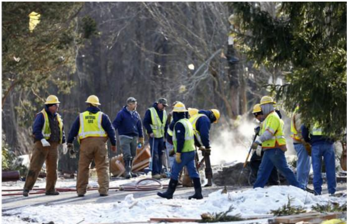
Utility workers inspect the damage following a blast in New Jersey.
