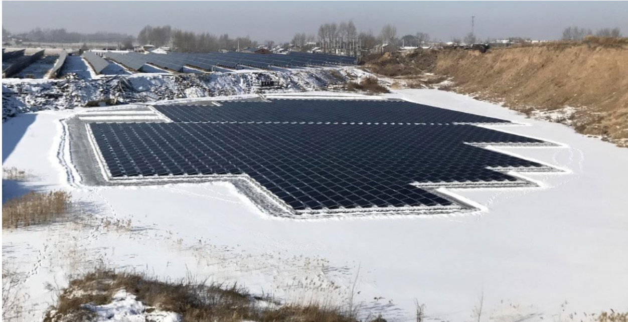
Figure 1: Floating Solar Installation in Bayan County, China
