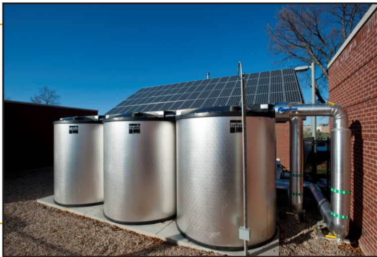
Thermal Storage Tanks & Solar Electric (PV) at the Academic Village Residence Hall
