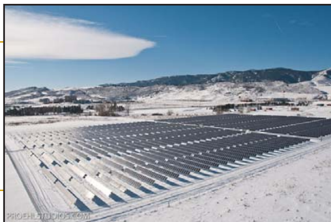
Two megawatt solar array at Chrisman Field
