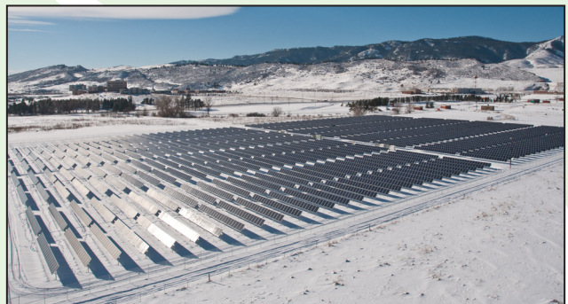
Two megawatt solar array at Chrisman Field
