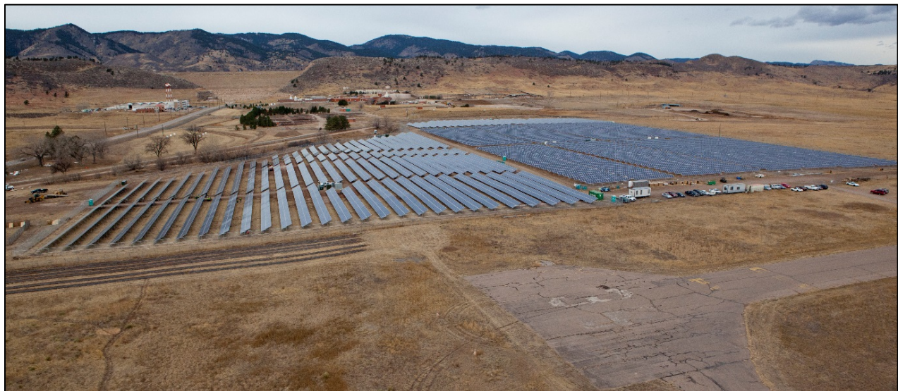
CSU Foothills Campus, Chrisman Field Solar Array – 5,300 kW
