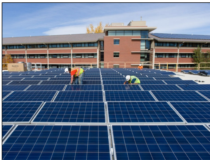
Solar array installed on Braiden Hall as part of the City of Fort Collins SP3 Solar Power Purchase Program
