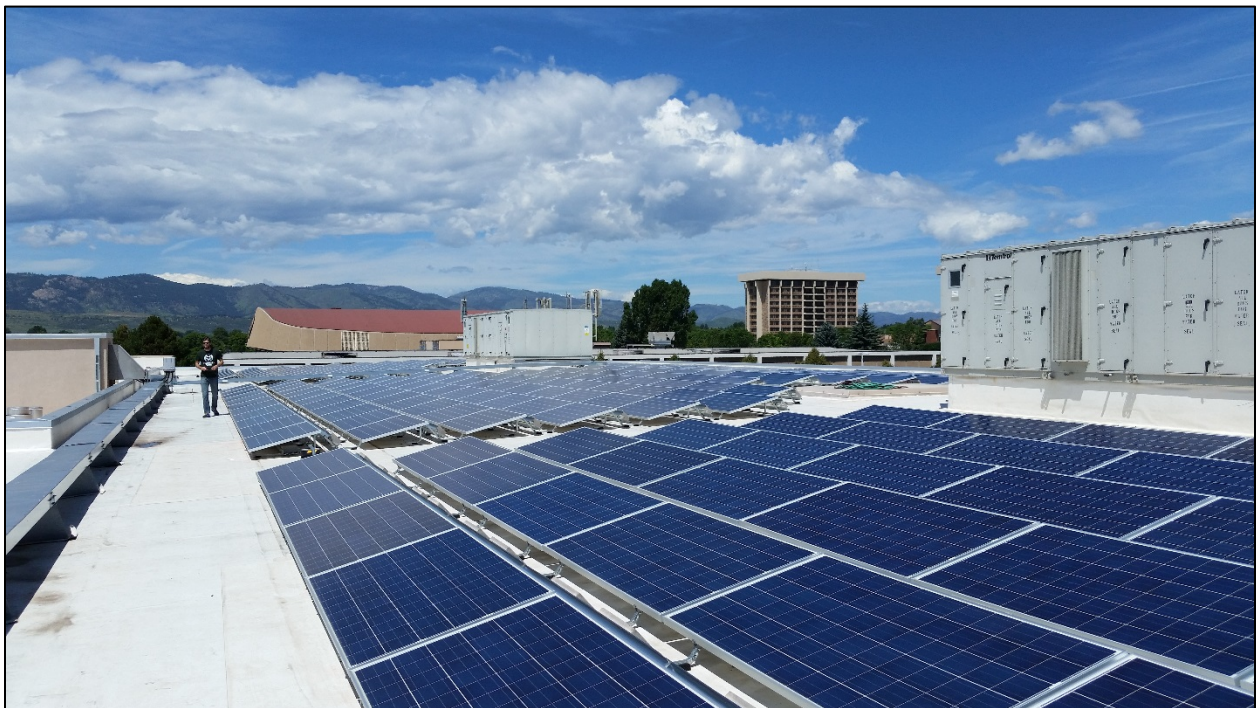
A 545 kW solar array located on the Student Recreation Center at CSU
