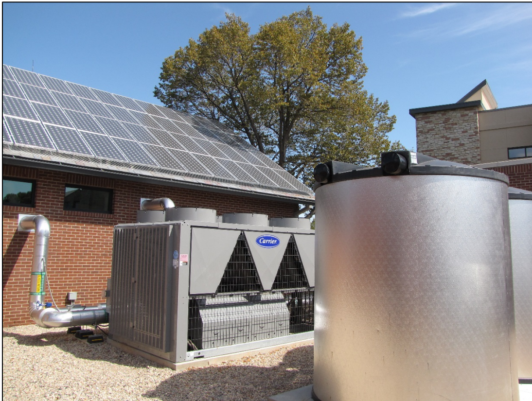
Thermal storage tanks & solar photovoltaic panels outside the Academic Village Residence Hall
