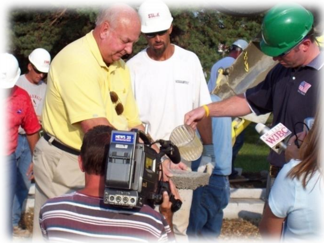
The porous nature of permeable concrete during a training session at the Hancock Field parking lot
