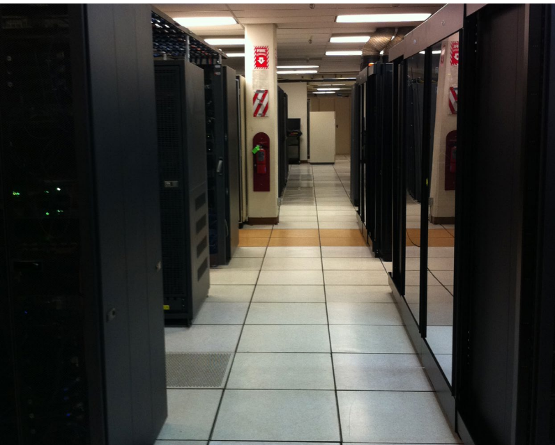
Photo: Data center end-aisle isolation
