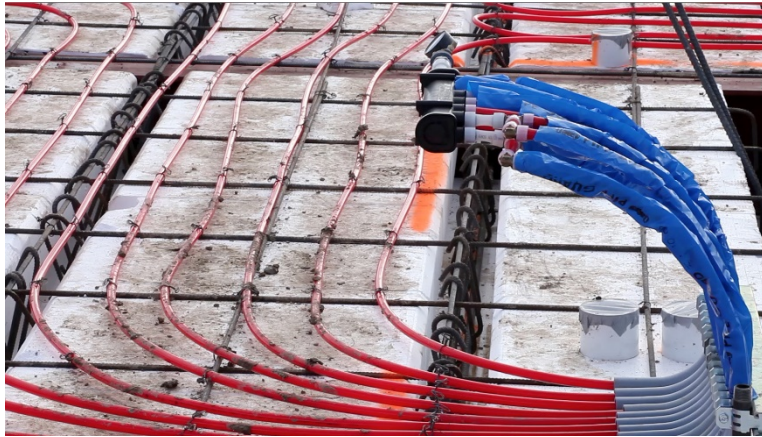
Figure 3. Example of Radiant Floor Installation on Main Level
