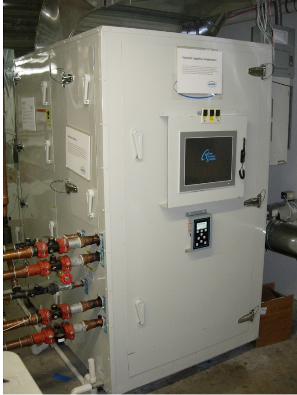
Figure 5. Air Handling Unit with Forced Air and Integrated Geothermal Heat Pump
