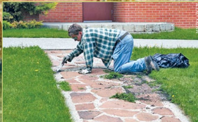
James Freeborn does maintenance work on the stone path between Wilson Hall and Danforth Park.
